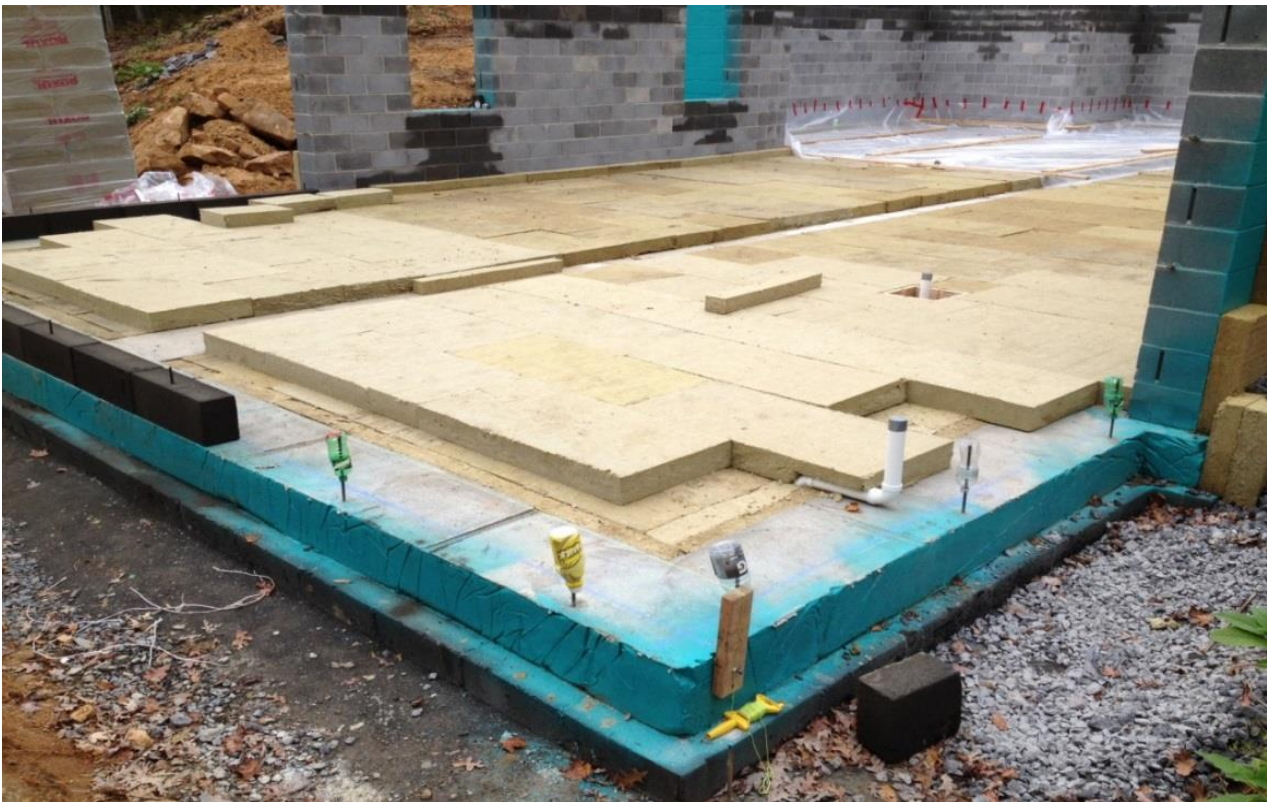
Installation photos provided by Michael Hindle, CPHC of Passive to Positive. Architect: Carri Beer, AIA of Brennan+Company Architects
